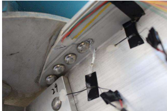
Fig.2 – Fracture at the joint flange.
