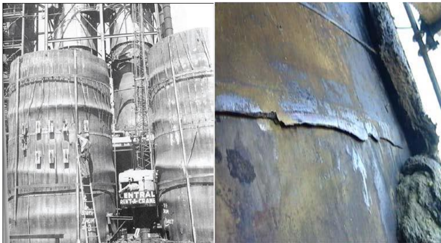
Fig. 1 Bulging and Cracking in Coke Drums
